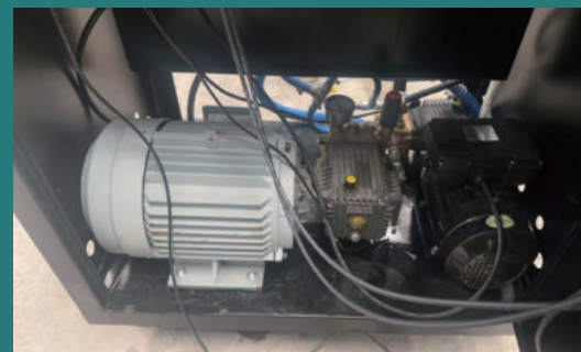
High pressure water pump&motor Pump used for foam proportioning
